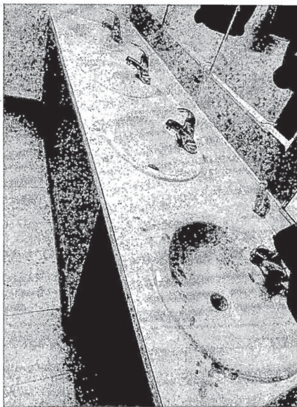
Dirty sinks at Ramp 23 bathroom of Louisville Gateway 10/2020.
